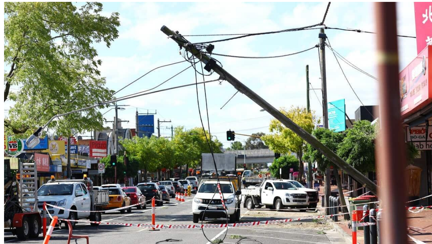
Storm damage 13 Feb 2024
